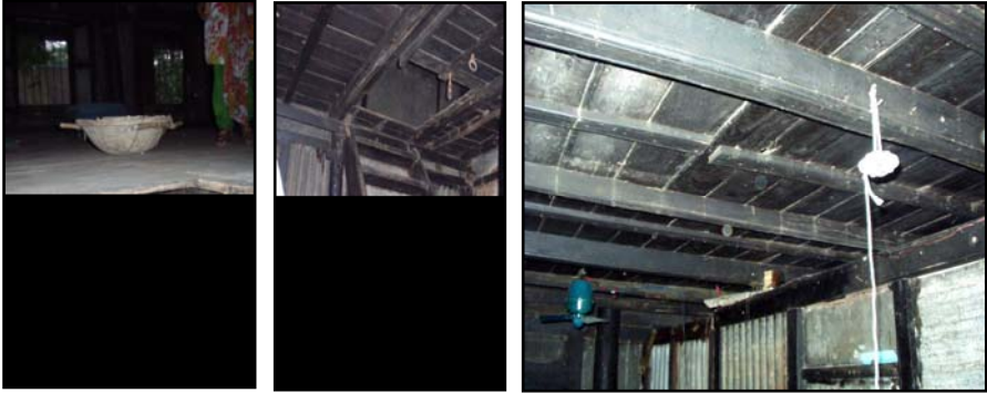
Figure 10: Thermal Data Logger position in upper space (right); Entry from indoor space to upper space (left); Wooden ladder for entering to the upper space (middle).
